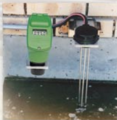
SHORTI SW controlling slur with ON/OFF Valve.
