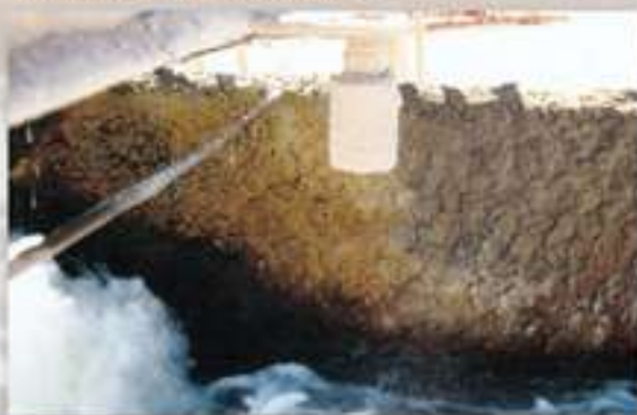
KAB 10 Covered with sludge measuring agitated surface
