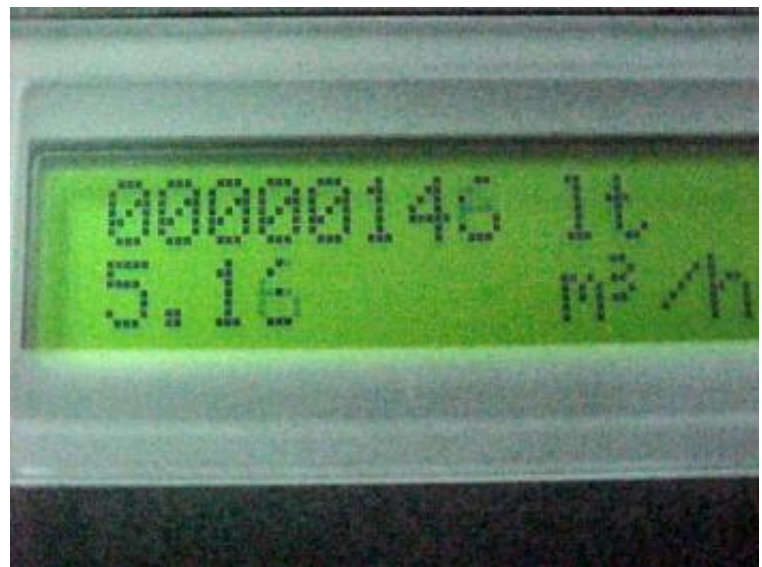
Flowrate and Totaliser
